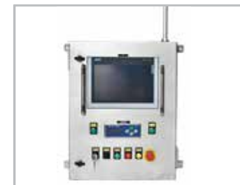
PLC based control panel as per PART11 CFR 21
